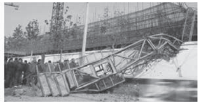
(c) 失稳的塔吊
